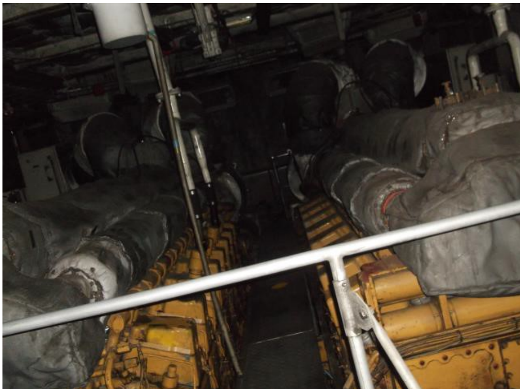
Inside engine room – (was reported in dry condition)
