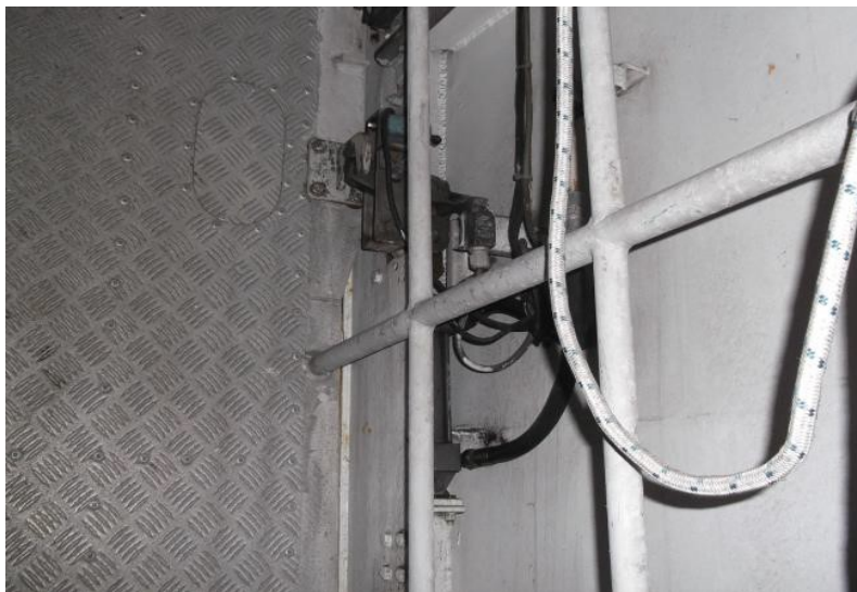
Close-up view of the hydraulic locking (fail safe) arrangement
