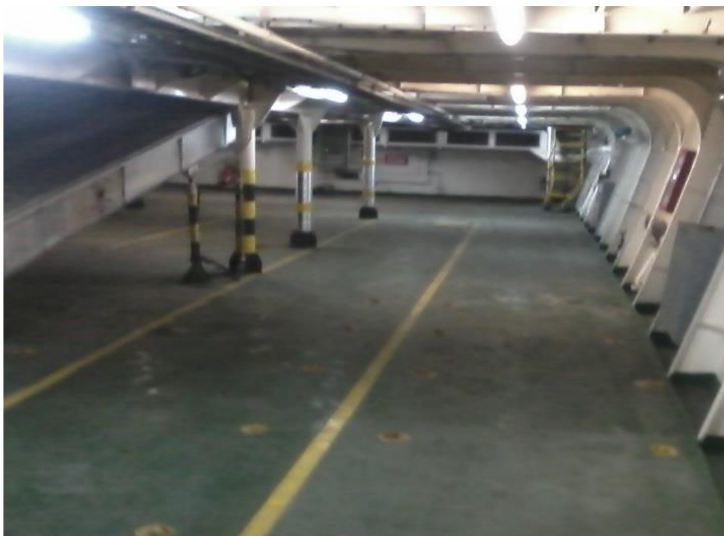
Vehicles deck– (was reported in dry condition) - Ro-Ro space (garage deck) visual inspection before sailing found it in good condition
