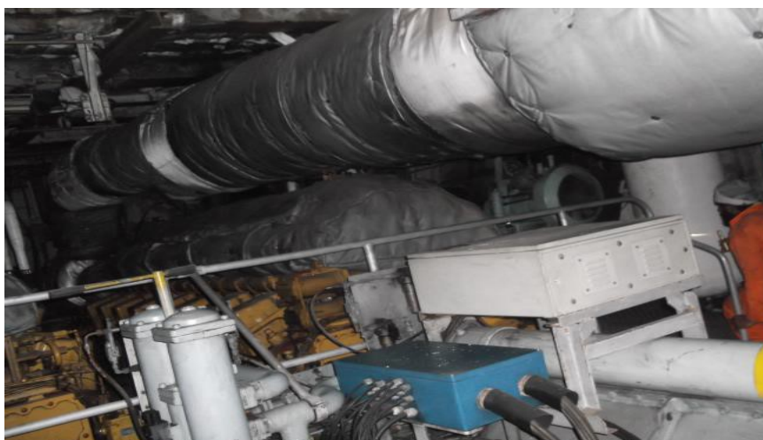
Inside engine room – (was reported in dry condition)
