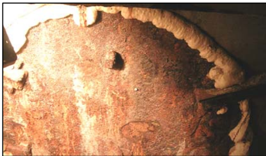
Figure 9: Steel plate and expanding foam blocking the access to the cargo hold
