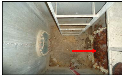
Figure 4: Ladder leading down the space. The access hole leading to the cargo hold is on the right-hand side
