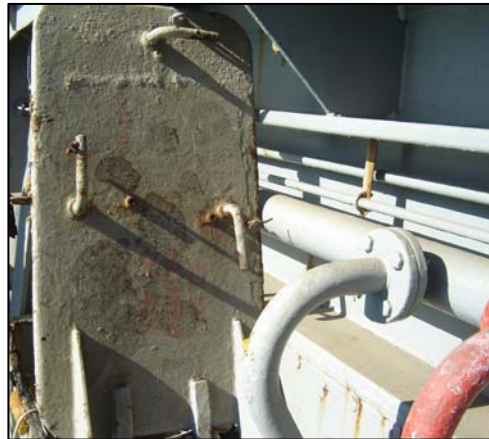
Figure 6: “Restricted Area / Zone” signs not painted on the access cover
